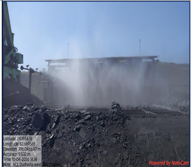
Fig:- Water Sprinkling Mechanism at Coal Crusher Unit
