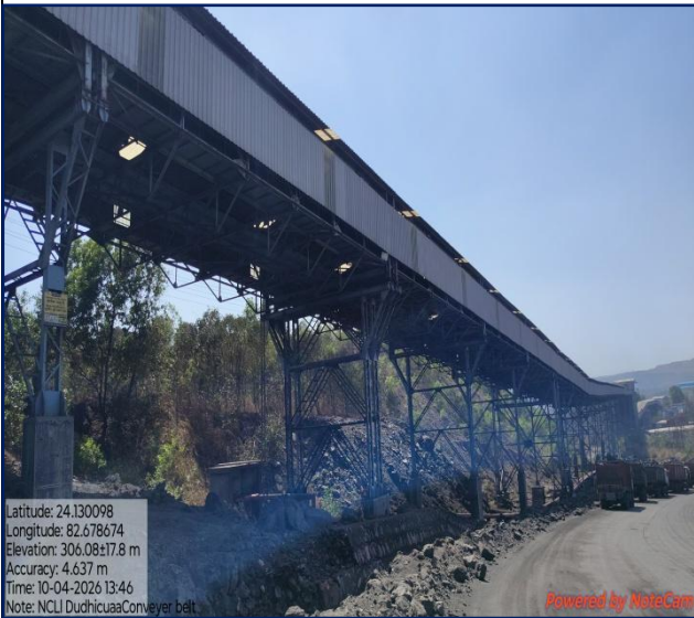
Fig:- Transportation of Coal through Covered Conveyer Belts
